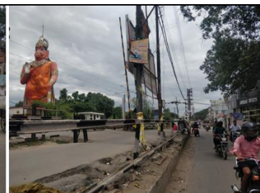
P1 Road Condition
